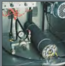
» BOILER INSULATION INOX AISI316
